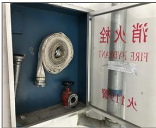
Photo of fire safety equipment 42 Fire hydrant.JPG
