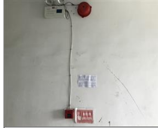
Photo of fire safety equipment 43 Fire alarm.JPG
