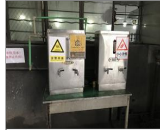
Photo of the sanitary facilities F31 Drinkable water.JPG
