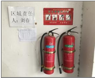
Photo of fire safety equipment 41 Fire extinguishers.JPG
